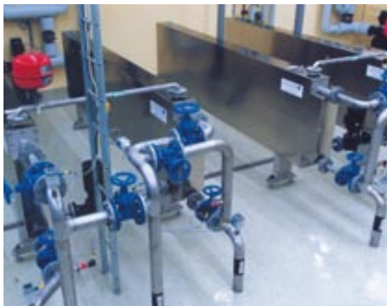
Two heat exchanger units sludge/sludge installed at Vimmerby wastewater treatment works.
